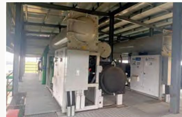
Online energy monitoring
